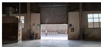
Emergency light not provided.jpg
